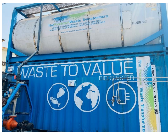
Photo of one of the TWT biodigester systems being installed in Freetown Sierra Leone
