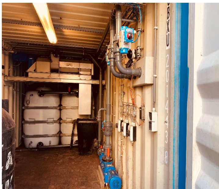
Photo of the digestate compartment of the biodigester system being installed in Freetown Sierra Leone
